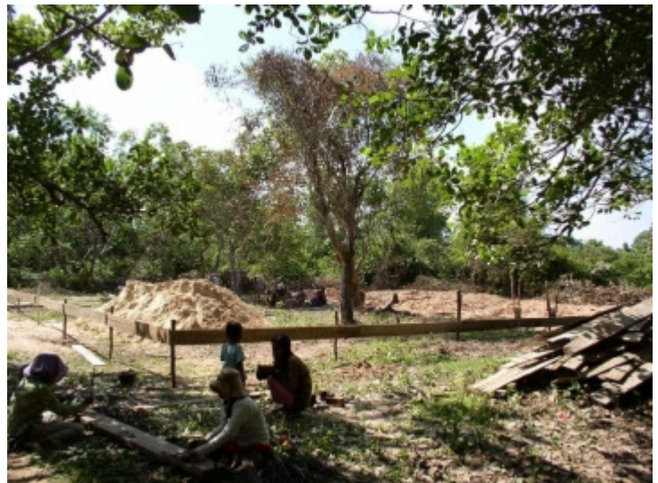
Trailblazer has finally received permission from APSARA Authority to proceed on the $24,000 Kindergarten school construction project. This is very exciting news! APSARA is the government office which oversees and must approve any development located within the ancient Angkor Temple areas. The Kindergarten site is adjacent to the Women's Development Center and Angkor
